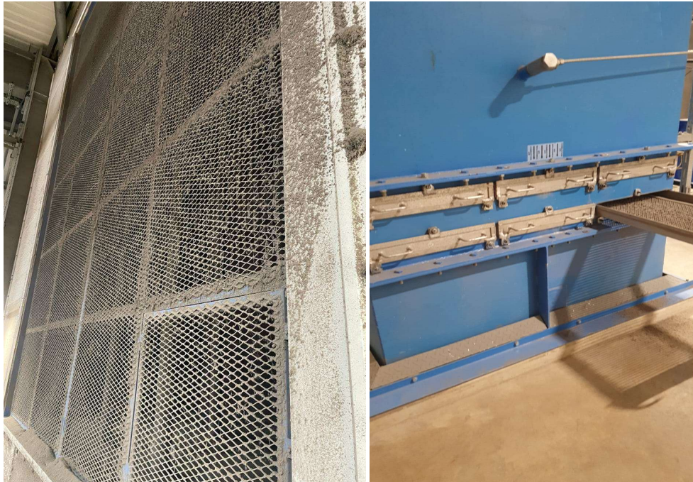
Figure 6-1 Primary air intake in the bunker hall & Figure 6.2 Primary air intake filters
